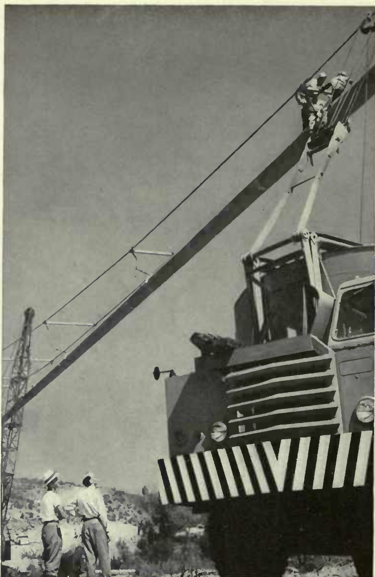
On its way from Texas to southern California, a natural gas pipeline is suspended at one point to cross a river.
